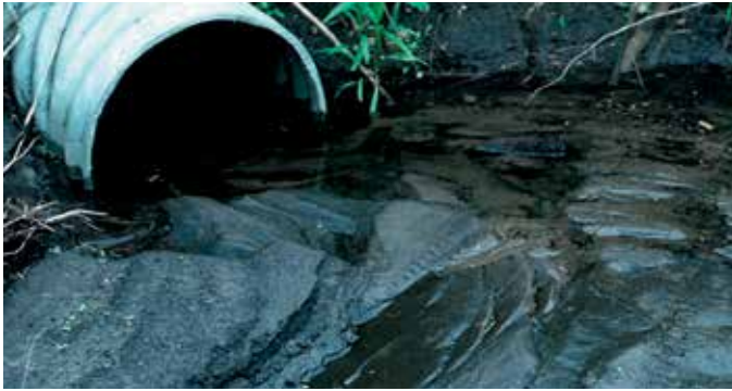
Sediments have filled up the opening of this drainage pipe that empties a stream into a lake.
